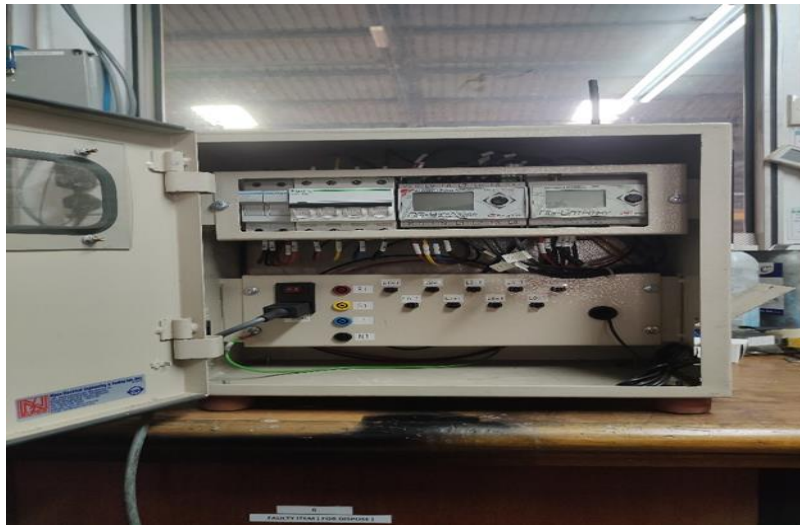
Figure 3.2: Energy monitoring device
